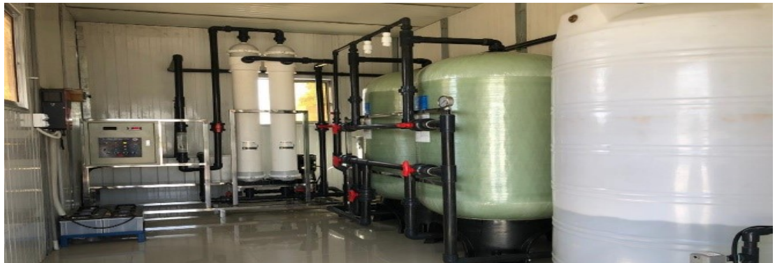
Solar powered UF plant installed in Karachi
