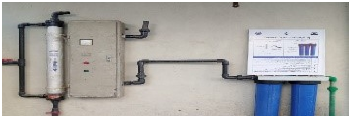
Drinking water filtration plant installed in schools
