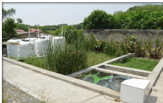
Picture wastewater recycling system for wetlands development
