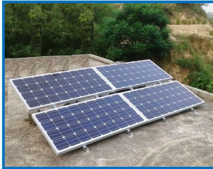
Figure 19: A view of the installed panels on the rooftop
