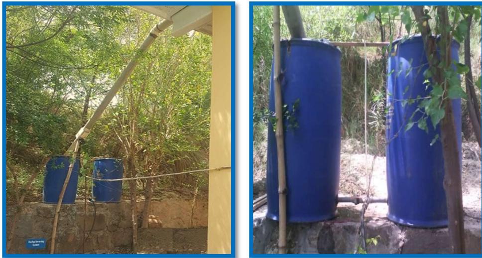
Figure 21: Farmstead rooftop rainwater harvesting system
