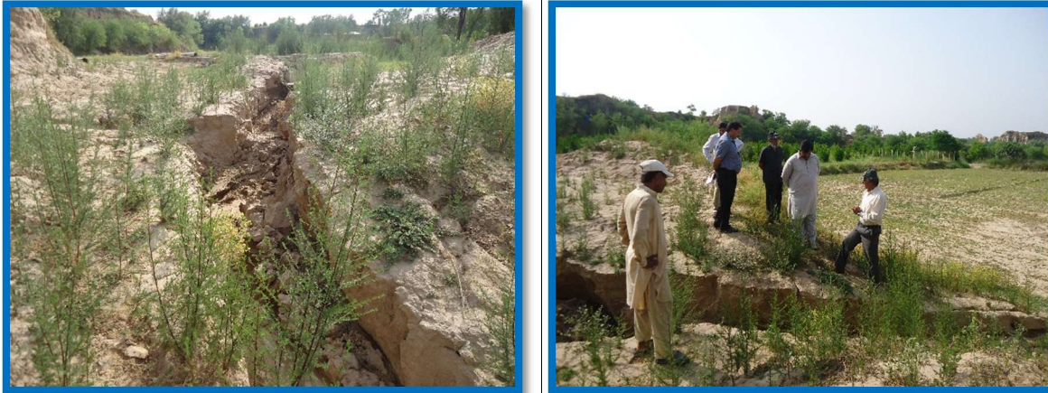
Figure 1: Soil erosion at the farm (2009)
