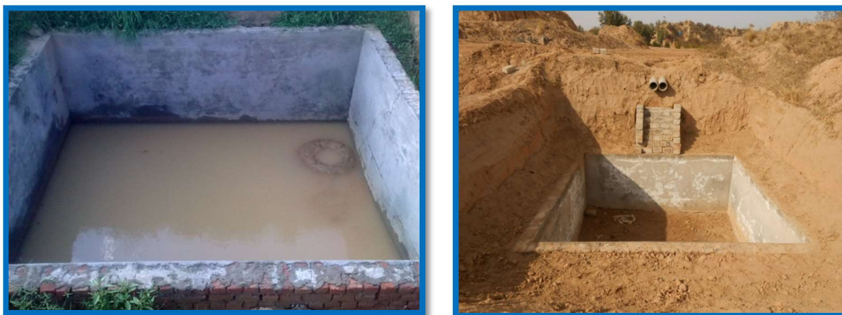
Figure 29: Stormwater harvesting ponds
