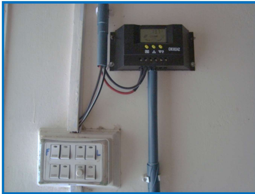
Figure 20: Charge controller regulating the battery charging rates
